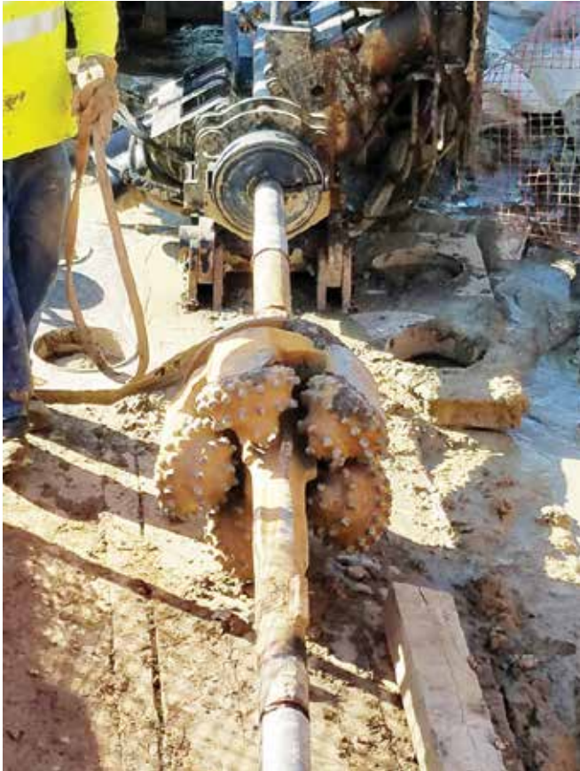
Thorough geotechnical investigations should be conducted before construction in all areas of planned HDD activity
